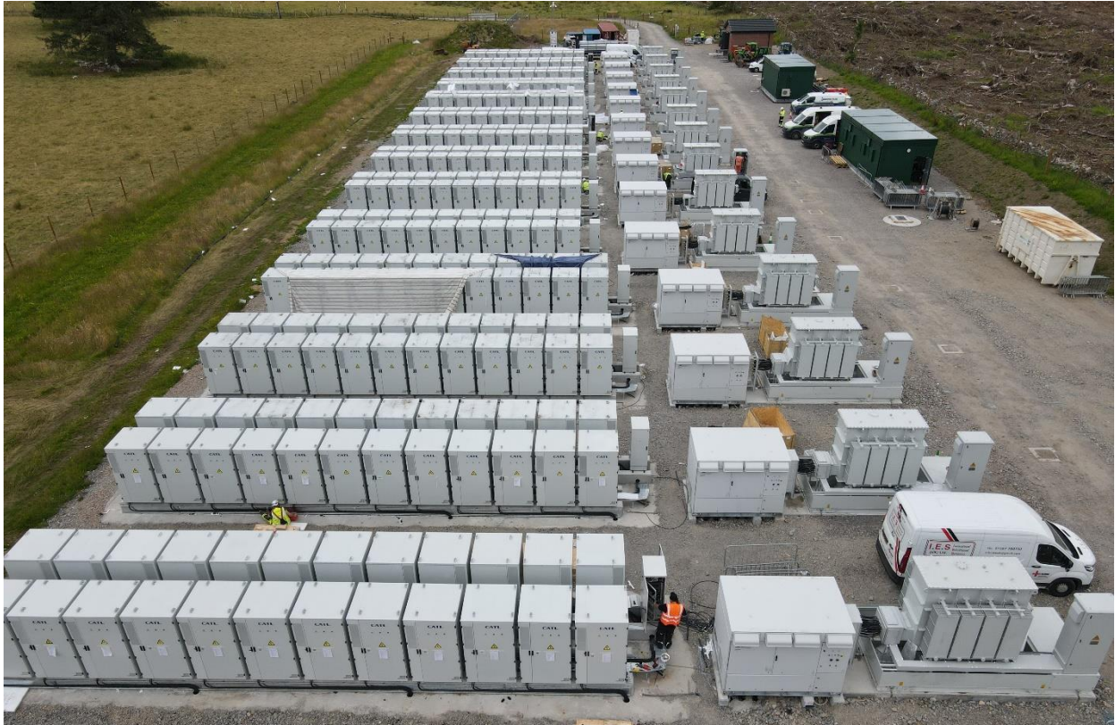
Figure 4 Typical cabined BESS and PCS
