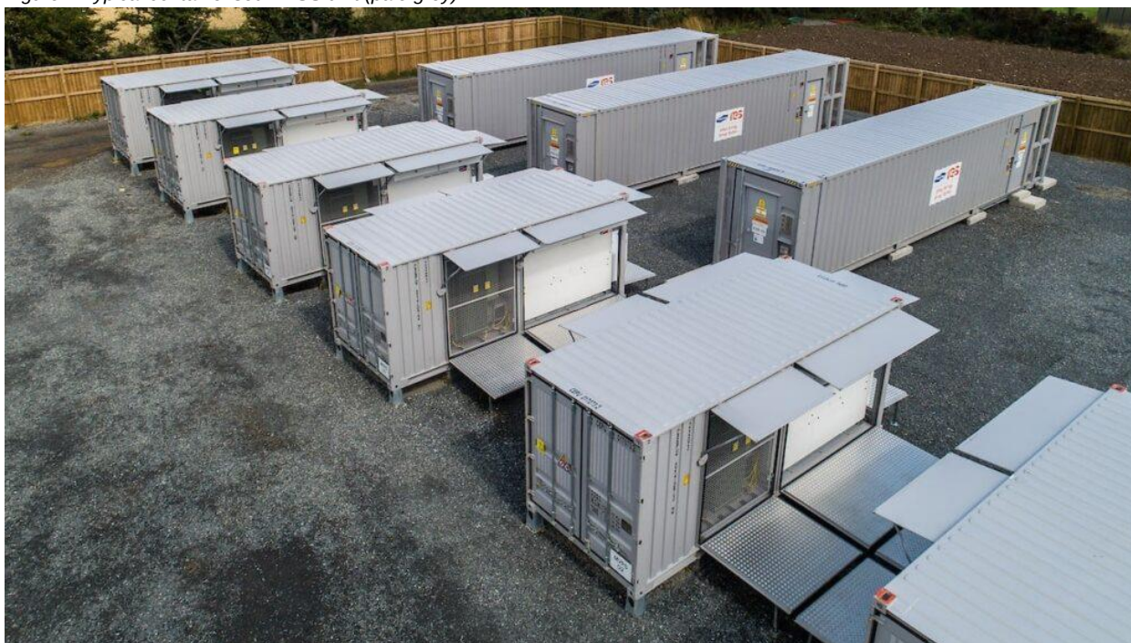
Figure 2 Typical containerised BESS units (right) and MV skids (left) in place (pale grey)
