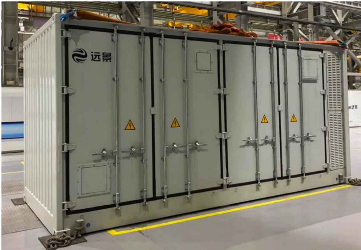
Figure 1 Typical containerised BESS unit (pale grey)
