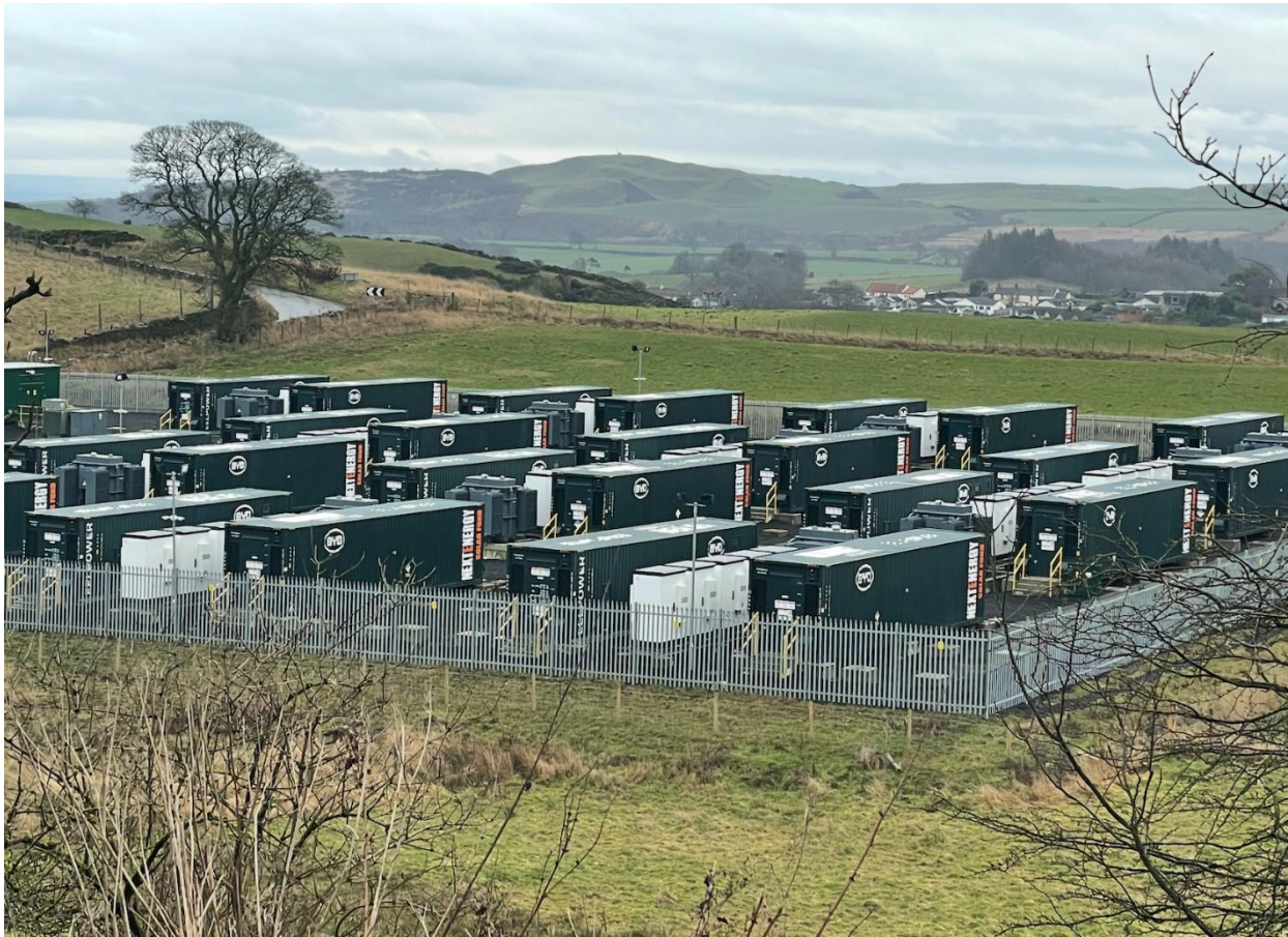
Figure 3: Typical containerised BESS units (dark green) and MV skids (white) in place
