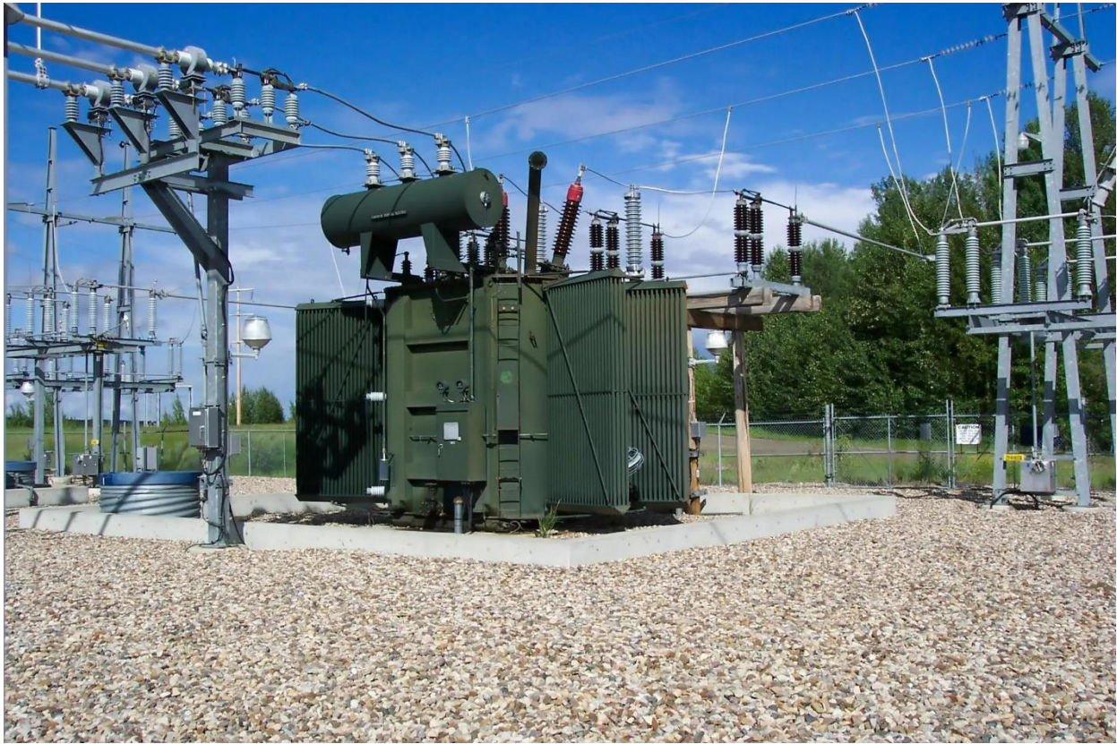
Figure 5 Typical transformer and switchgear
